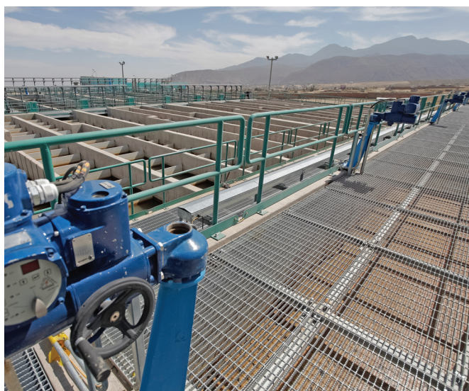
Wastewater treatment in Arequipa. Studies are under way to make the sludge from tanning waste available for use in fertiliser. This is one of a series of circular-economy initiatives under way already in the Peruvian city's leather cluster. Credit: David Huamani Bedoya/Shutterstock
