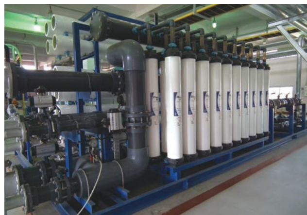
After tertiary treatment, remaining suspended solids are removed by ultra filtration.
