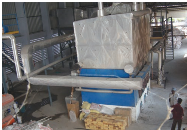
Wood and biomass steam generating plant.
