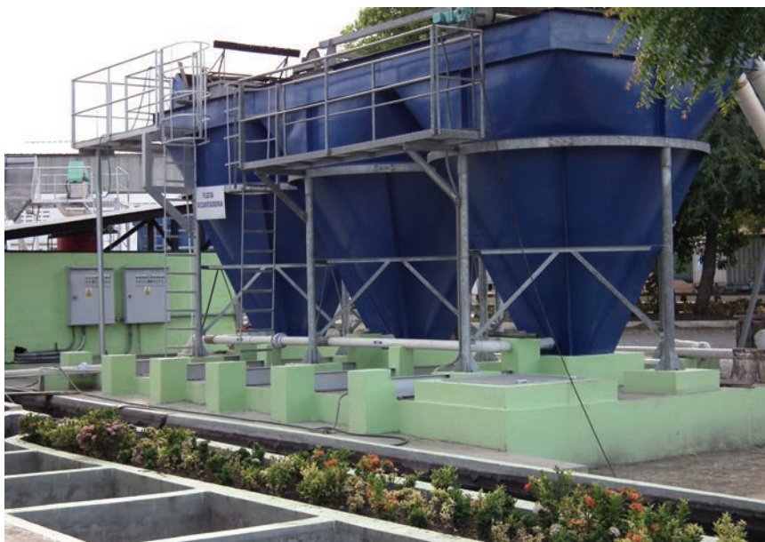
Modern effluent treatment plants have transformed the global industry to the extent that a tannery today can be sited in an urban area and the local population is largely unaware of the tannery on their doorstep. This photograph shows part of a primary effluent treatment system installed at a tannery within the city of Santiago, Dominican Republic.
