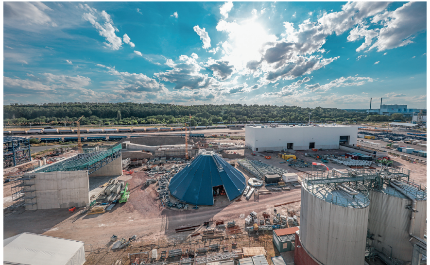
The new UPM Biochemicals plant at Leuna in Germany this summer. It will be operational before the end of 2023.
