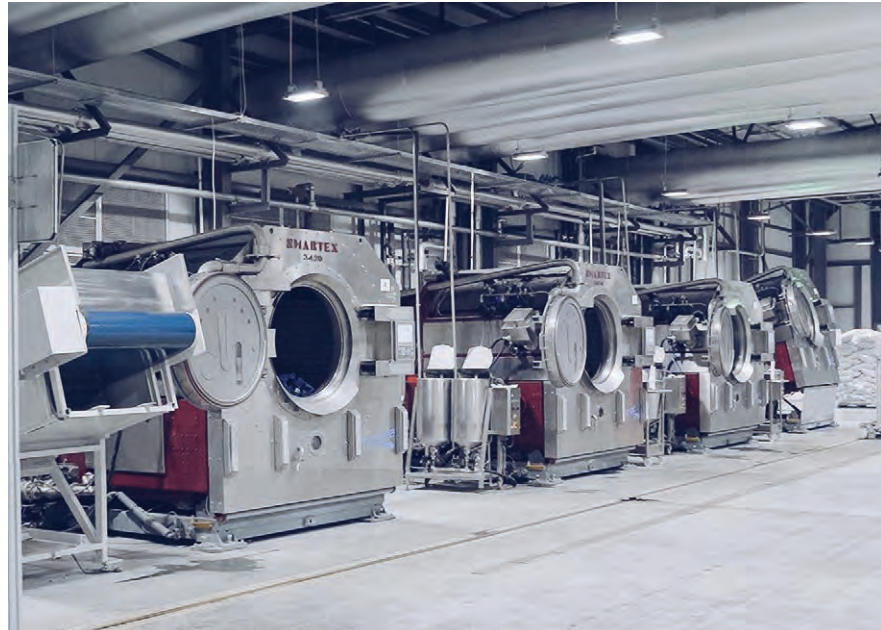
Eurotay, part of Turkish group Taypa, has been operating a highly automated facility in Serbia since 2019.
